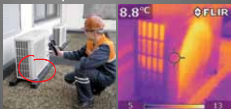
Check-up of a heat, ventilation and airconditioning installation quick and easy.
