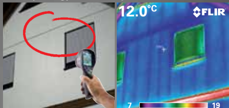
The thermal inspection locates missing insulation in the wall. To avoid further energy loss, missing insulation must be installed quickly.
