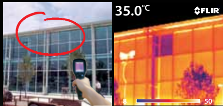
The thermal inspection reveals an incorrect window installation. The coating is placed on the inside instead of the outside of the window.
