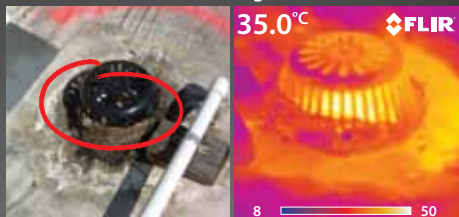
The thermal image shows water leakage in the roof.
